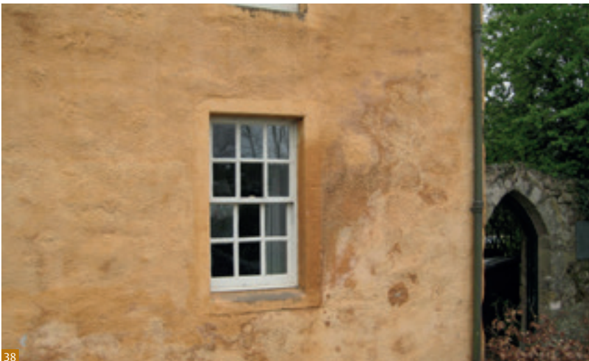
Fig. 38 Patchy appearance of limewash requiring maintenance.
