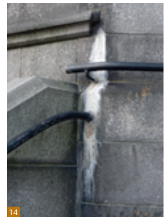
Fig. 14 Example of streaking caused by excess free lime content on the lime mortar.
